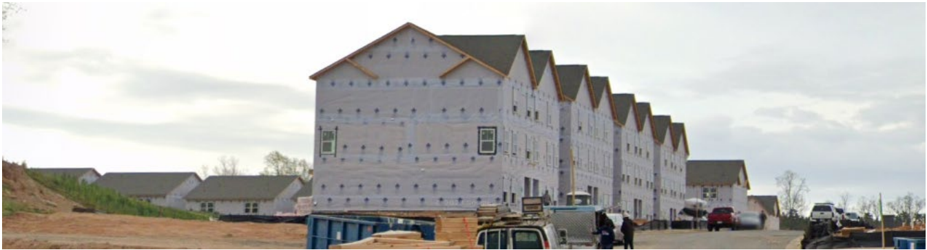
North of the site are single family attached and duplex dwellings under construction as Phases 2-4 of the Blu South development.
