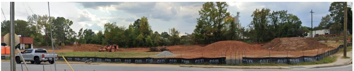
Streetview of construction underway to the east of the site at the intersection of State Street and Gesco Street. This site will be a mix of multifamily residential, single family attached residential, and commercial uses.
