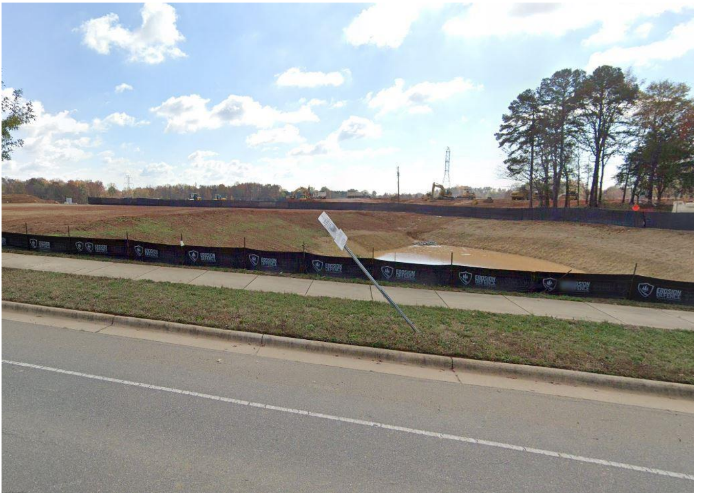
View of the multi-family development, currently under construction, located on Johnston Oehler Road southeast of the site.
