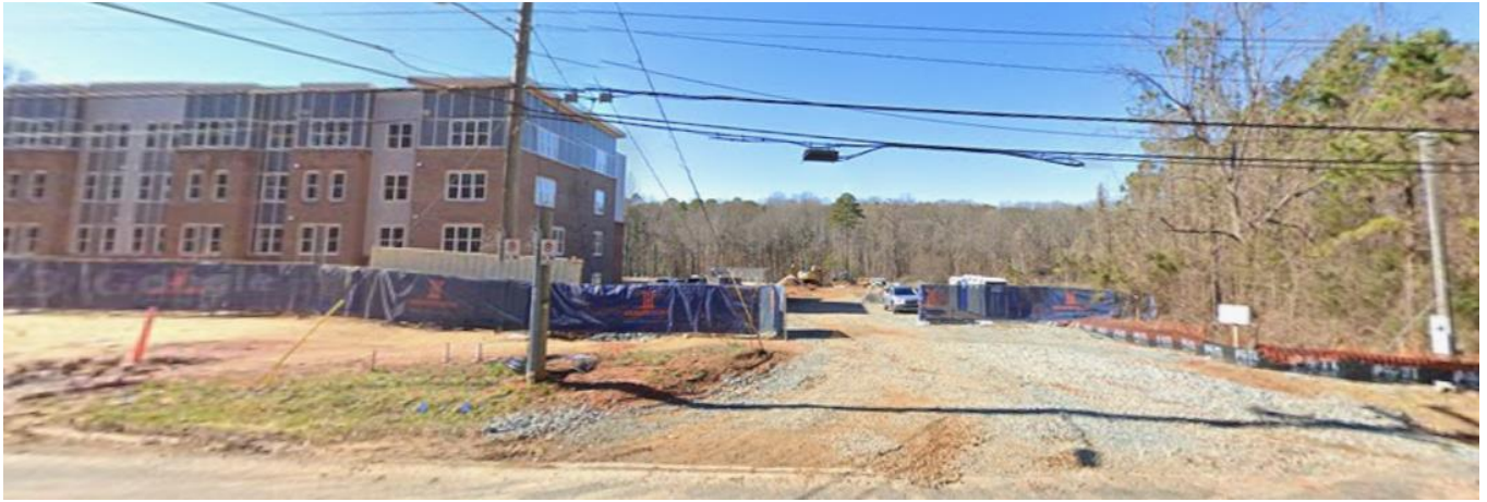
View of Banner Ridge Boulevard under construction. The site will gain primary access from an extension of Banner Ridge Boulevard. The building shown to the left of Banner Ridge Boulevard is a multi-family stacked development, under construction when the image was captured, zoned INST(CD) (Institutional, conditional).
