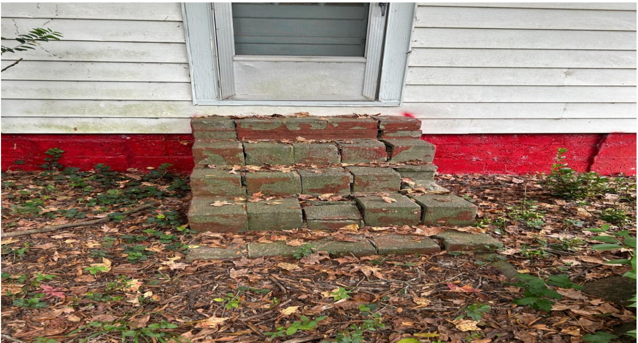
Rear entrance (missing mortar; unstable steps)
