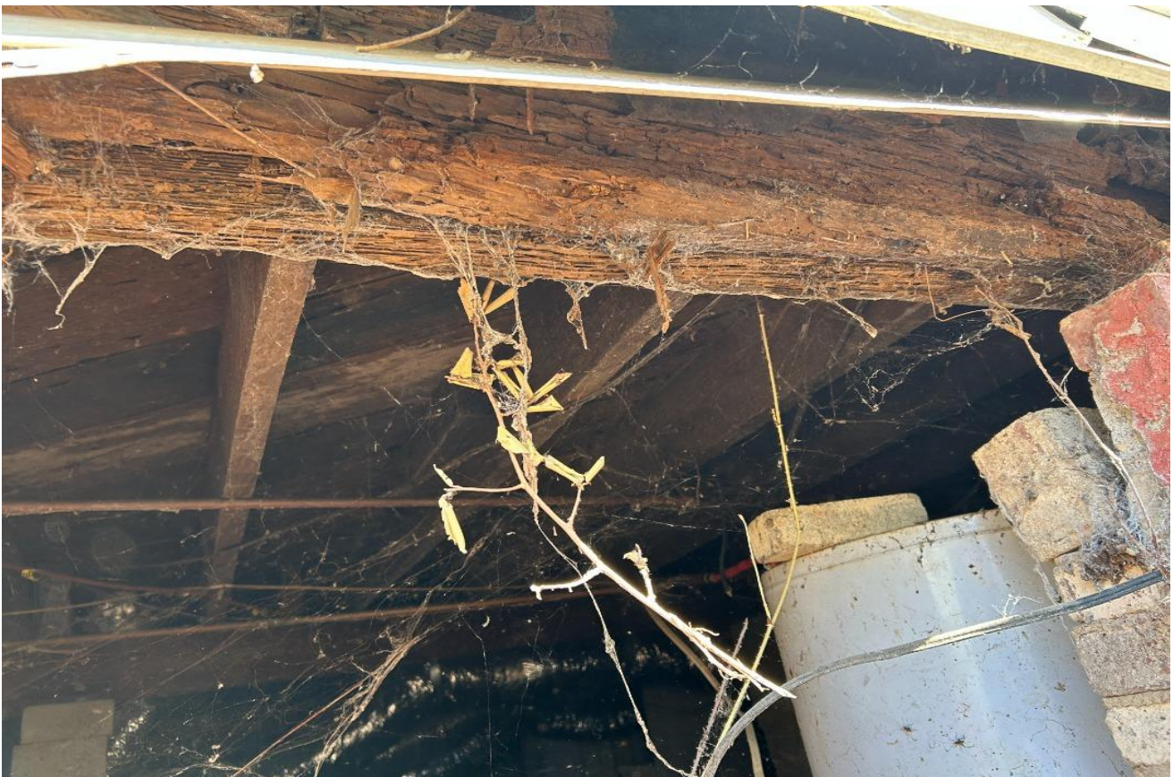
Crawl space (decayed sill)
