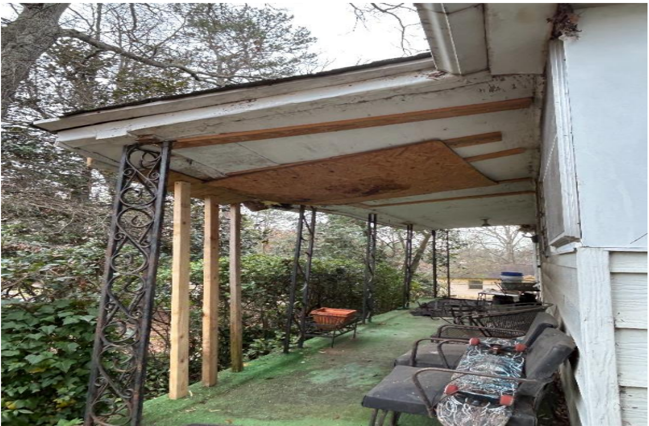
Front porch (collapsing)
