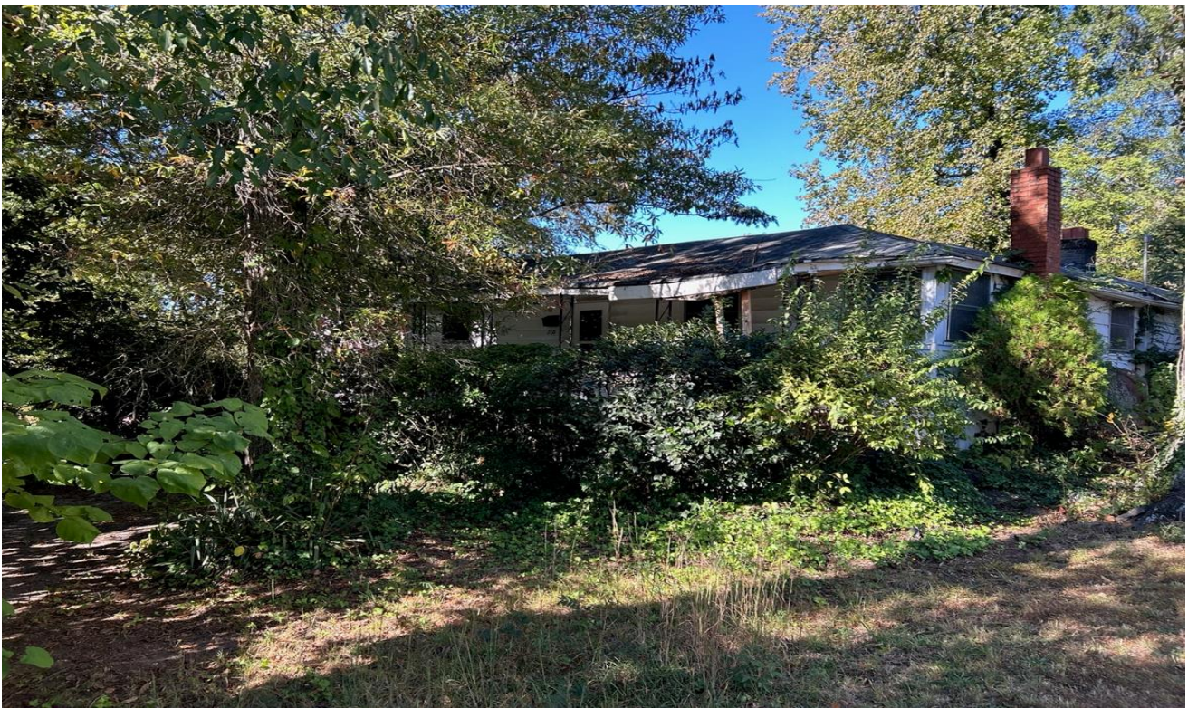
Front exterior from street (front porch collapsing)
