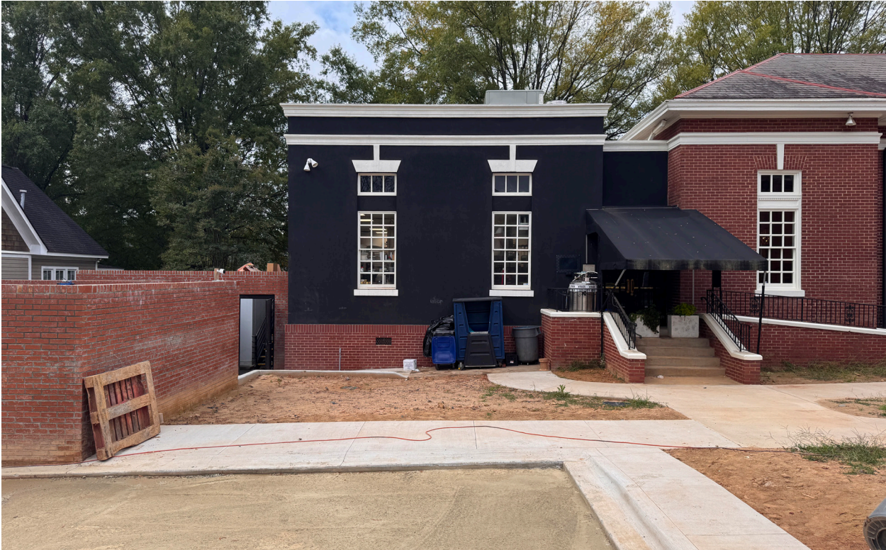
5. Looking southwest, view of a previous addition at the rear of the building.
