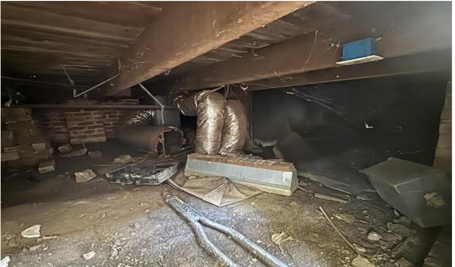
Crawl Space (missing heating equipment)
