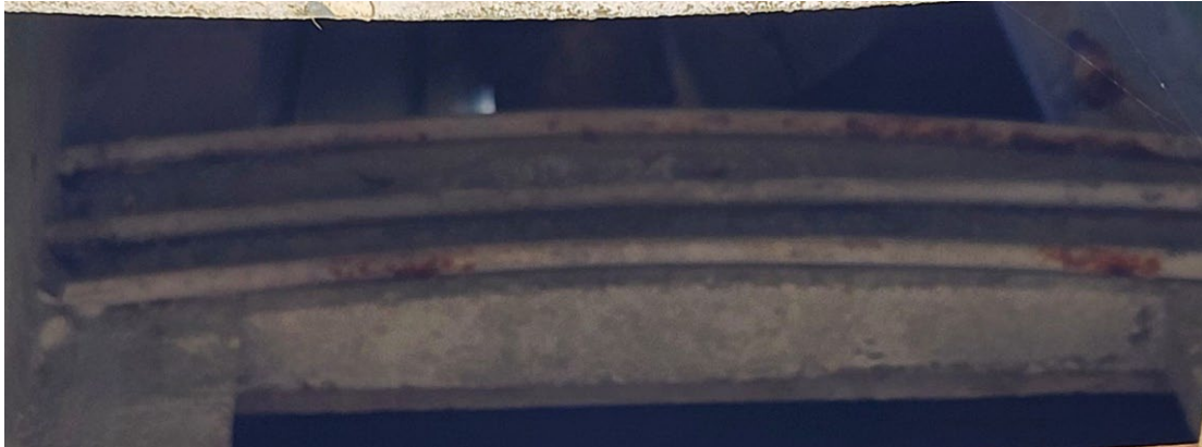
Above: One of the concrete lintels within the north silo's front elevation poured concrete frame that spans the silo's continuous door. Note the reinforcement hoops.
