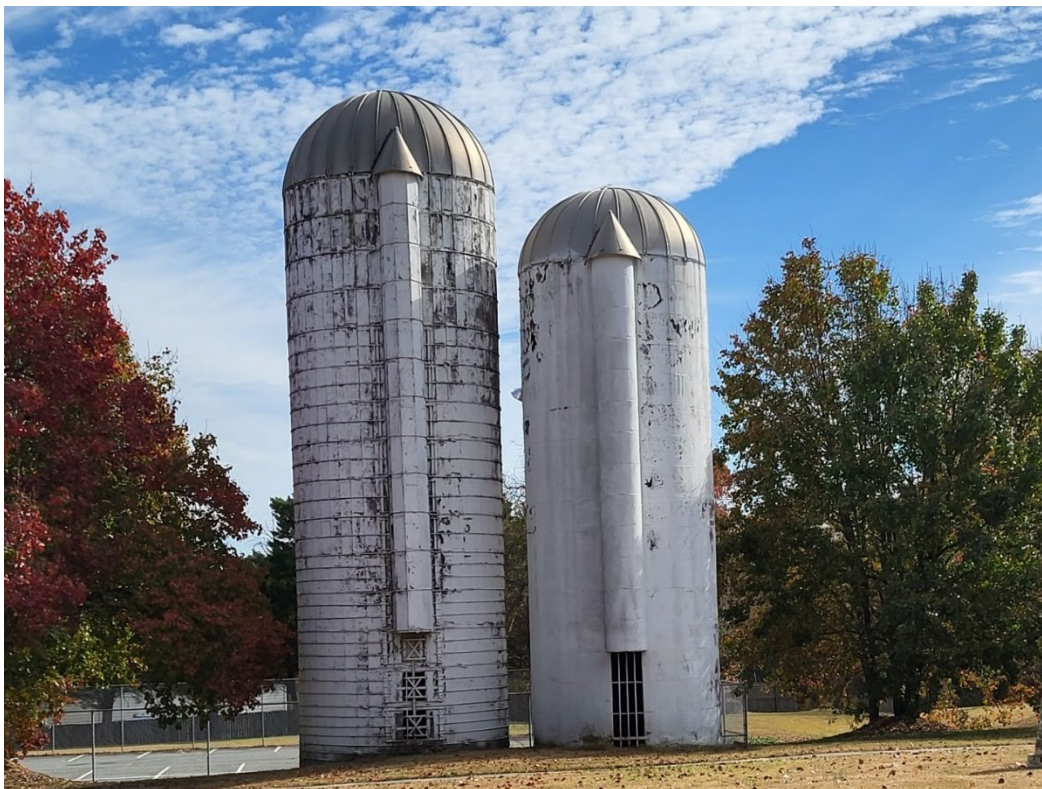
Faires Farm Silos – Front/West Elevation. North silo on left, south silo on right.
