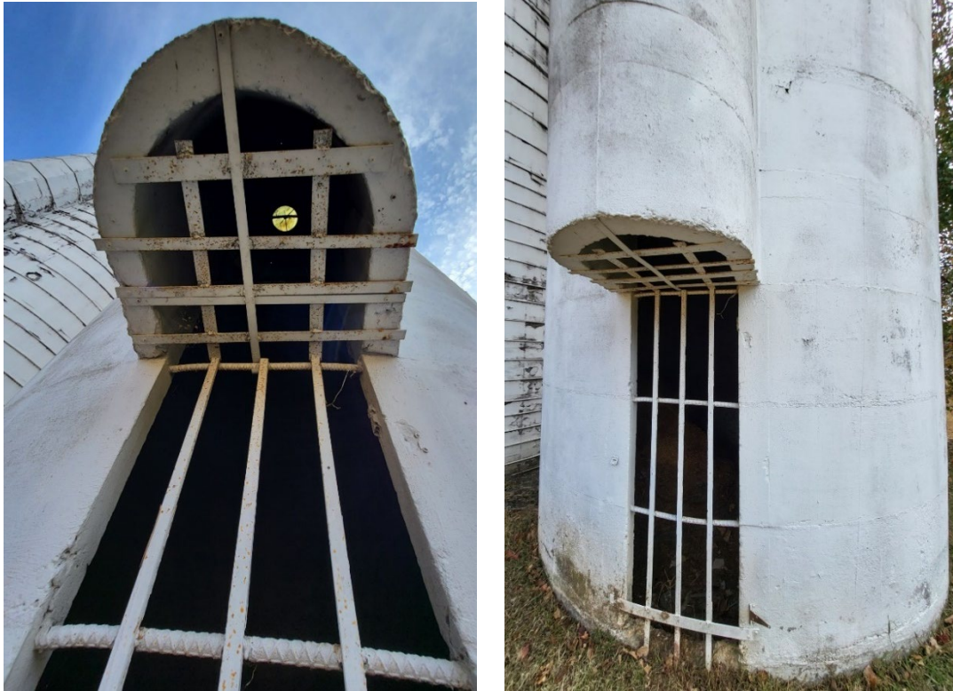
Chute opening (left) and bottom portion of continuous door (right), both on the south silo's front/west elevation.
