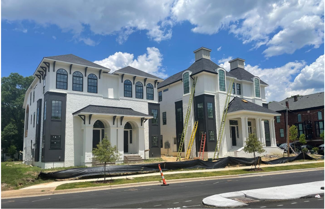
Figure 6 The duet units under construction in June 2017. They are located on the western portion of the property along Parkwood Avenue.
