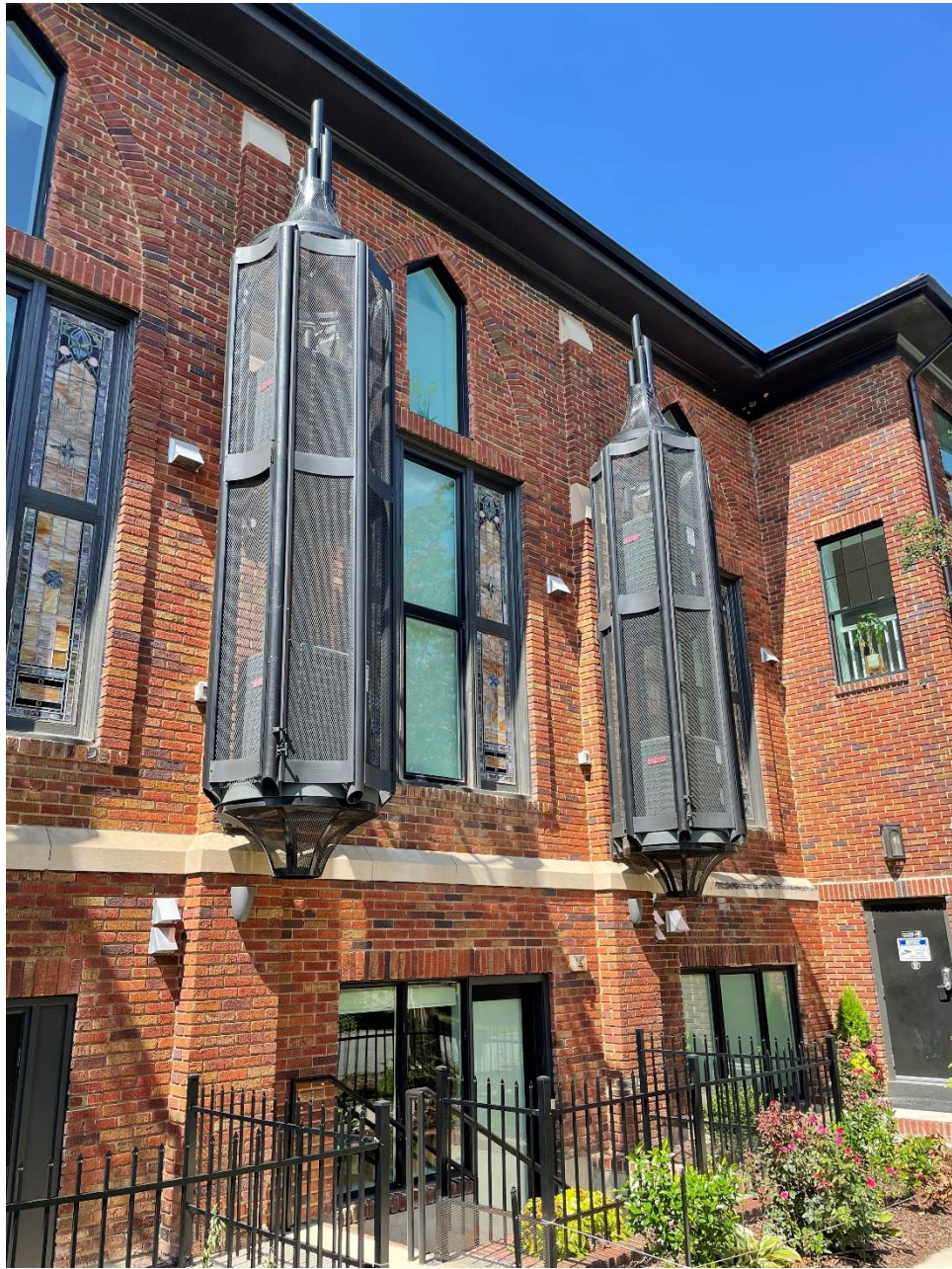
Figure 16 Typical heat pump surround at east elevation, 2023.
