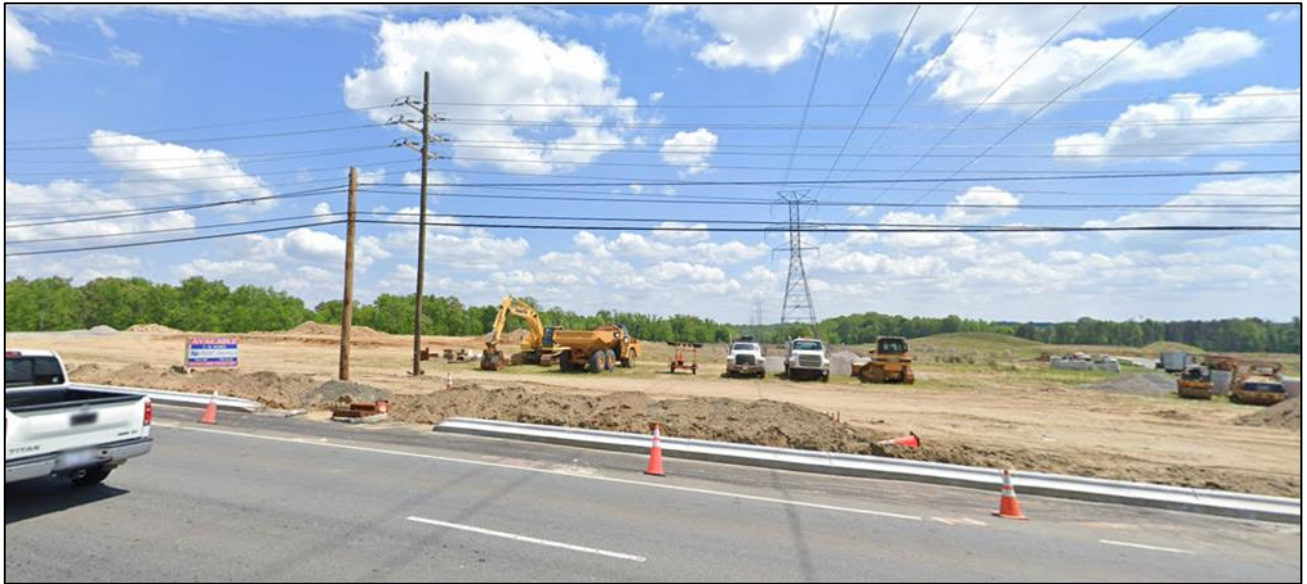
The site is vacant and being cleared and graded for construction. A Duke Energy transmission traverses the site.
