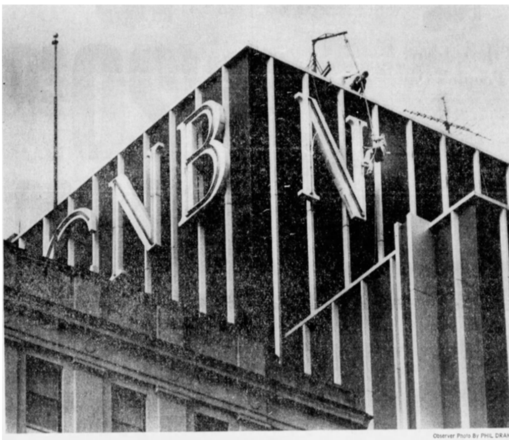
Sign Art Inc. employee installing NCNB Sign, The Charlotte Observer , Credit: Phil Drake
