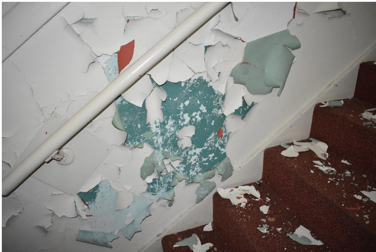
A variety of previous paint colors are visible under the chipping paint in the west stairwell.
