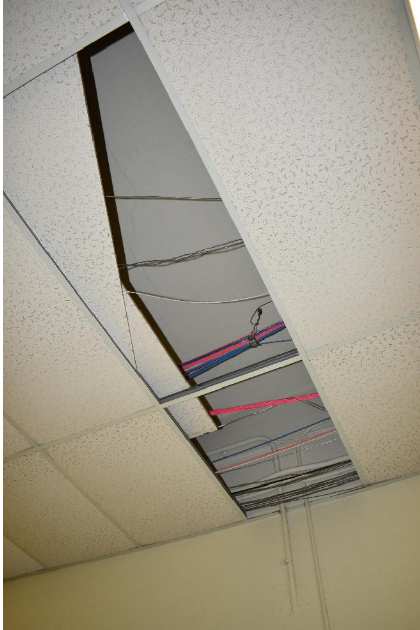
Plaster ceiling visible under acoustic tile ceiling in the first floor hallway of the original 1925 building.
