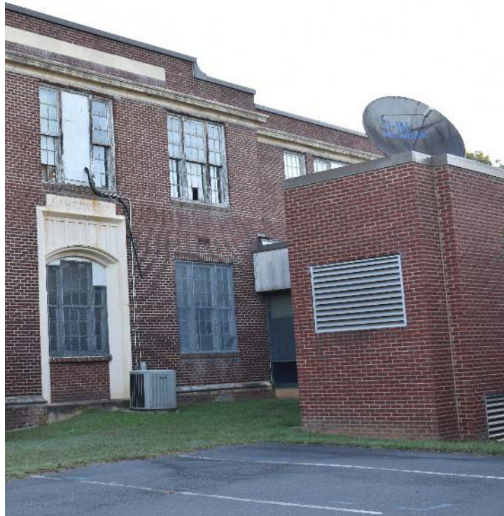
South elevation of the 1925 original building with west elevation of 1970 library/administrative addition.
