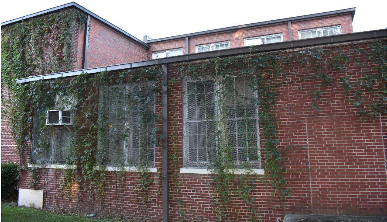
East elevation of 1948 cafeteria addition and second-floor classroom added to the back of the auditorium.
