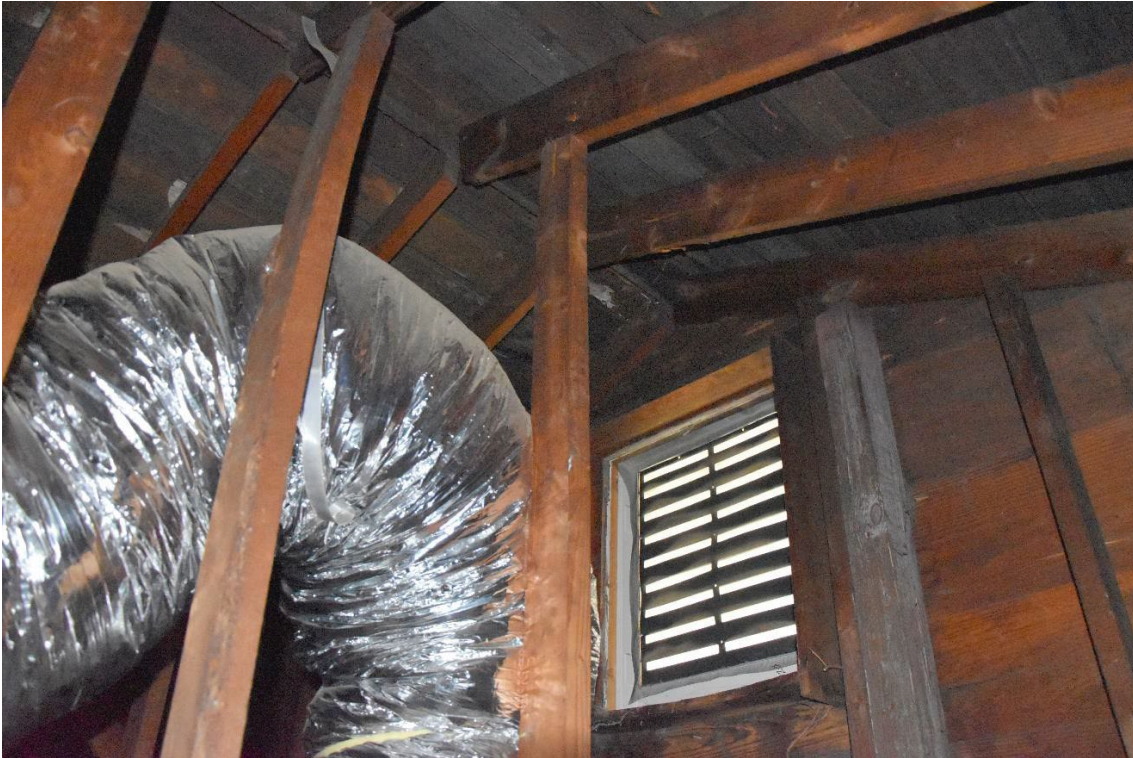
Figure 20 Visible are the roofstructure and louvered vent in the exterior wall of the left elevation looking east.
