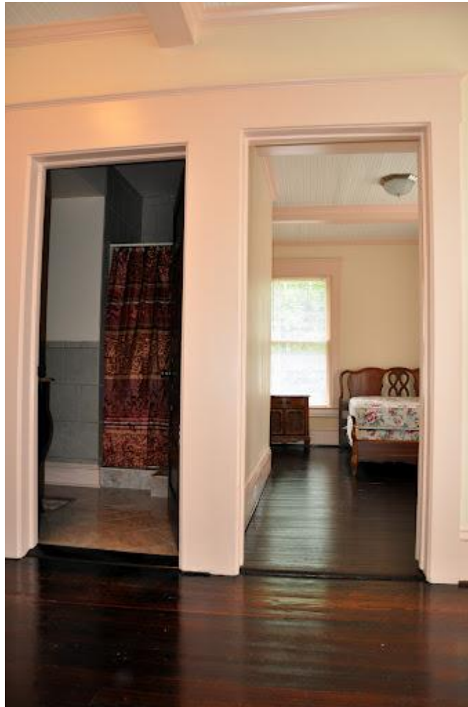
An original door opening (right) in comparison to a new door opening (left) in the second story.
