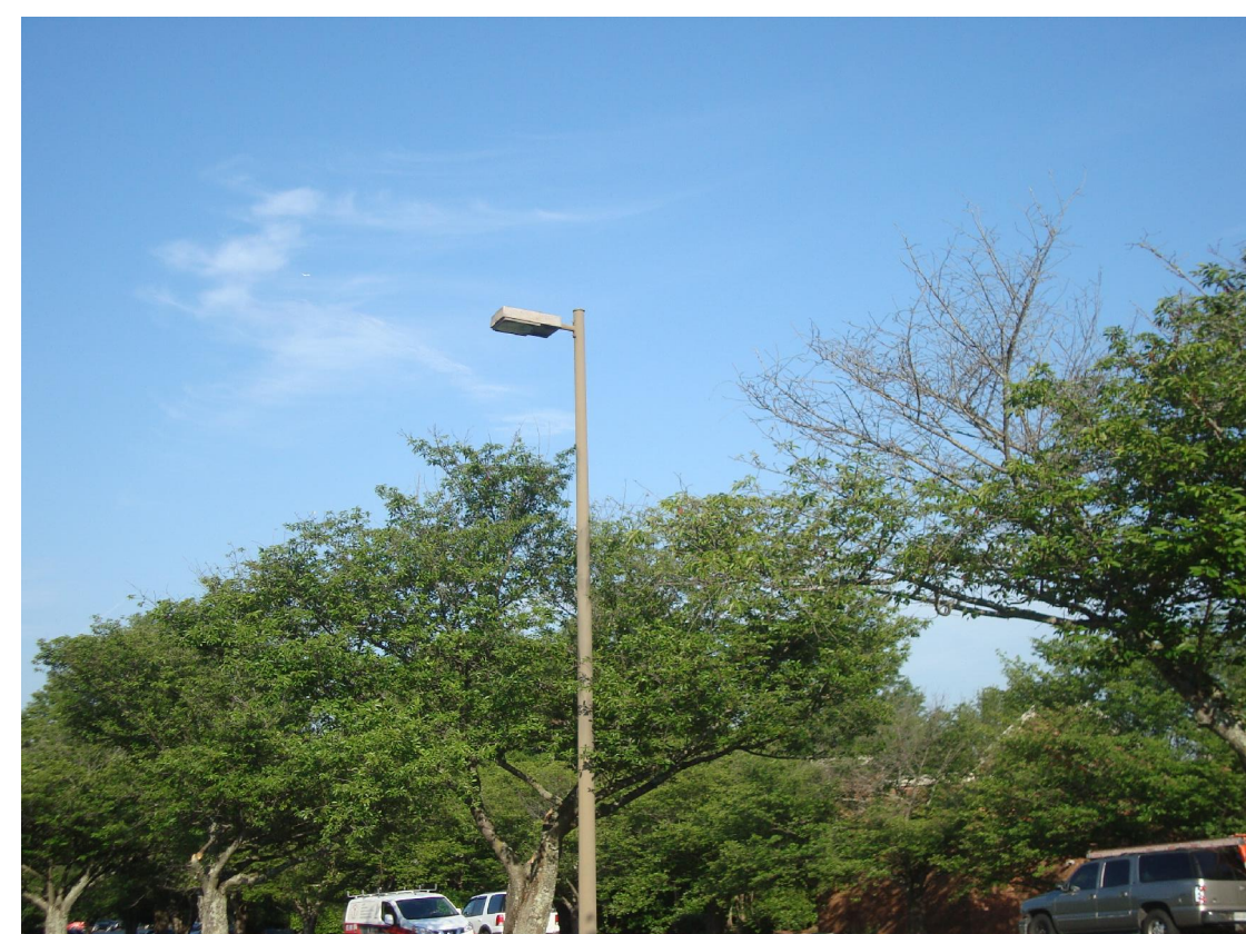
EXISTING SITE LIGHTING
